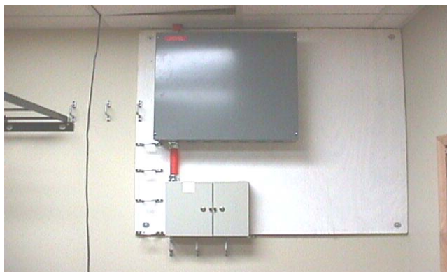
Photo 31: 24 port Wall Mount Enclosure and Spare Fiber Enclosure.
