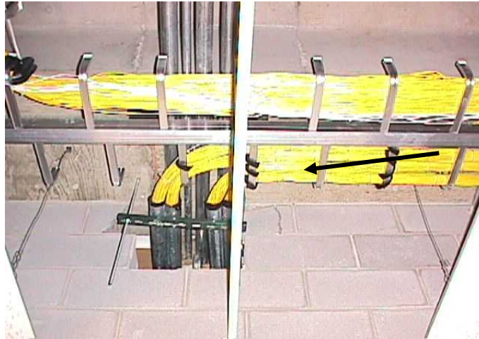
Photo 13. Cable tray installed above drop ceiling.
