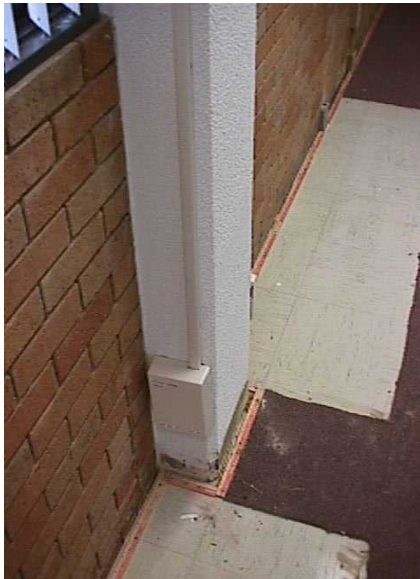
Photo 18: Example of exposed raceway application. Attached to the pillar.
