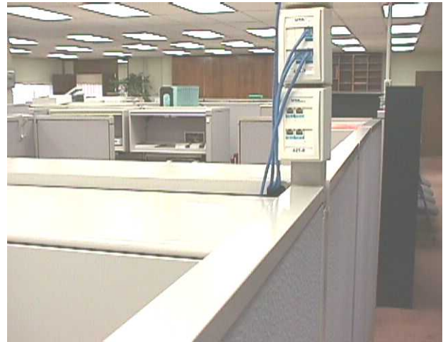
Photo 22: Example of one-piece single gang junction box (P/N JB1IW-A) mounted to a power pole to feed the top caps of modular furniture. Junction boxes are faced with PANDUIT Brand Executive style Mini-Com faceplate (P/N CFPE6IWY).
