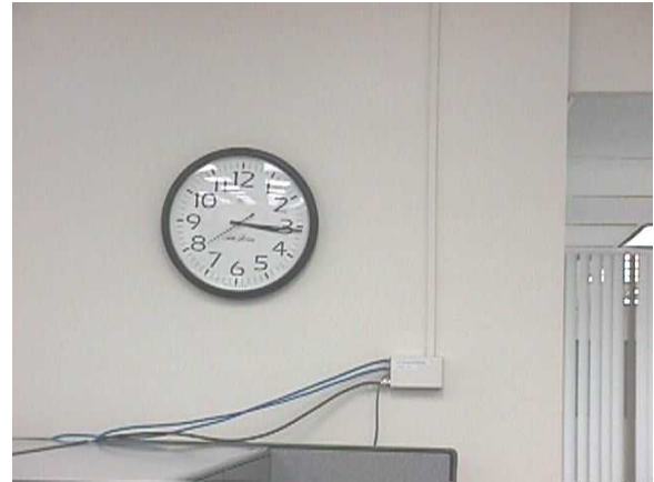
Photo 19: Example of exposed raceway application. Mounted on a non-hollow wall above the level of the modular furniture.
