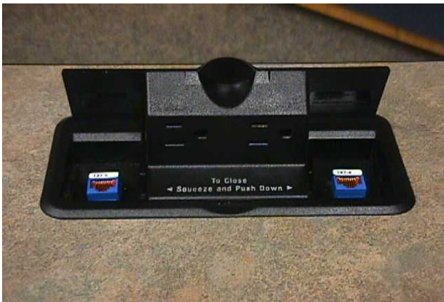
Photo 29: KI PowerUp Module with Panduit Keystone jacks installed.
